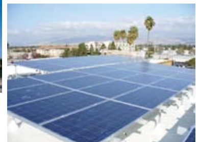
The project's photovoltaic array is highlighted in this photo
